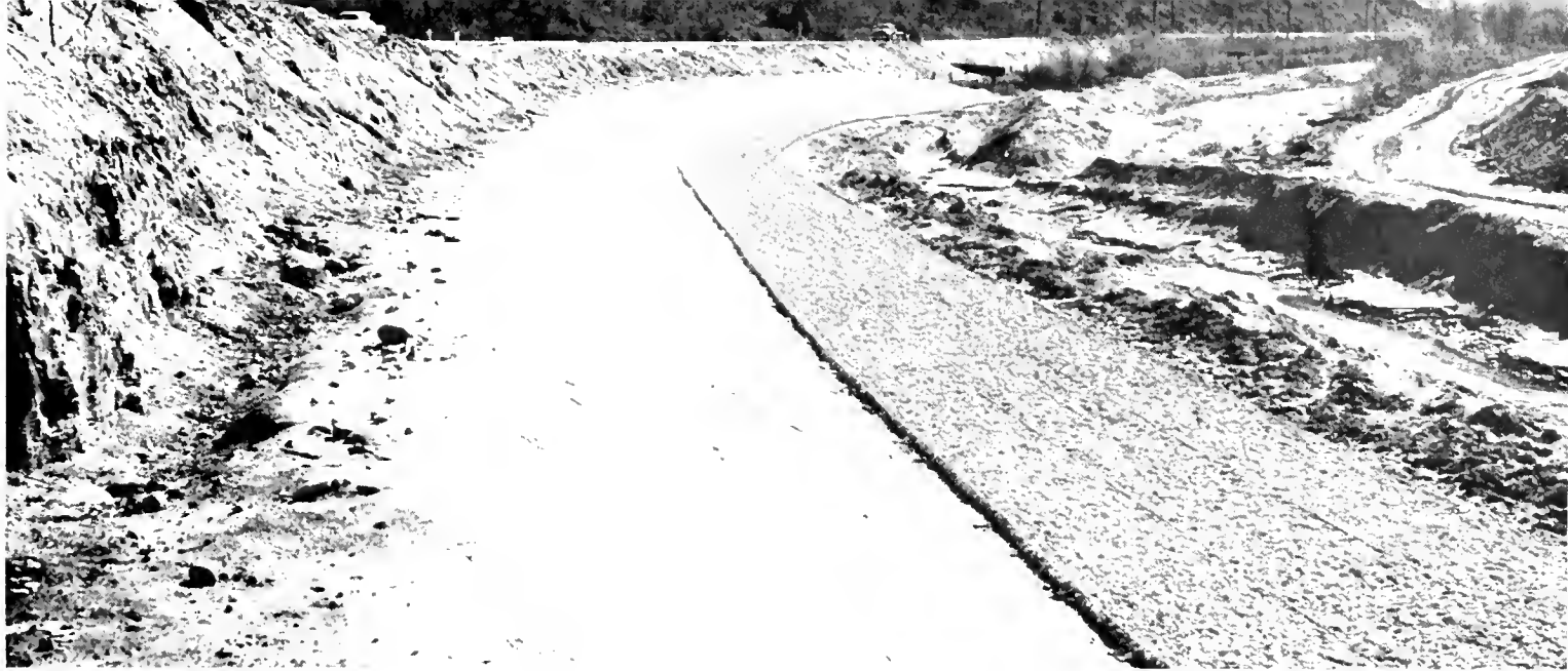
Portland cement concrete revetment on 1½:1 slope 10 inches thick with rock and wire mattress 14 feet 6 inches wide
